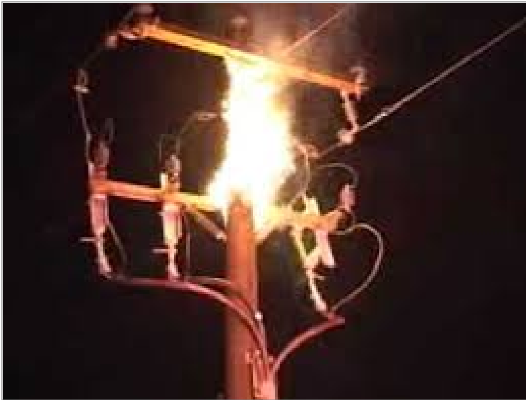
Photo 2: Pole top fire
