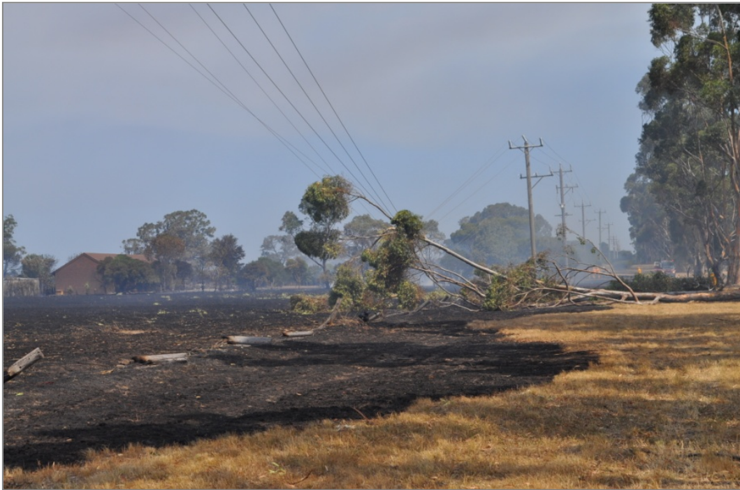
Photo 1: Hazard tree located outside of the easement fell into 66kV electric line and started a fire.
