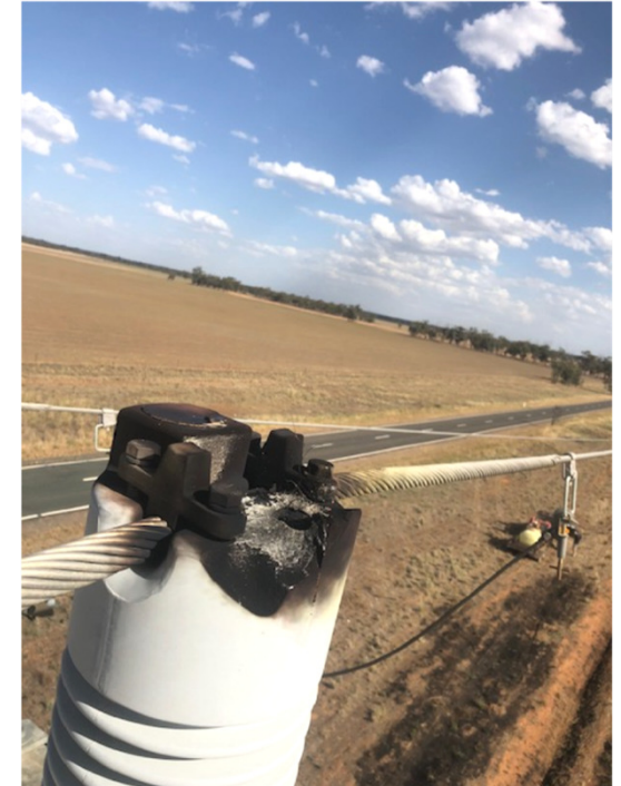
EHK024 fault 3 rd February
